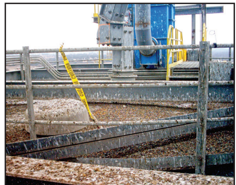
Bird droppings can harbor disease, parasites and other harmful organisms. They are corrosive and will damage surfaces if not cleaned.
